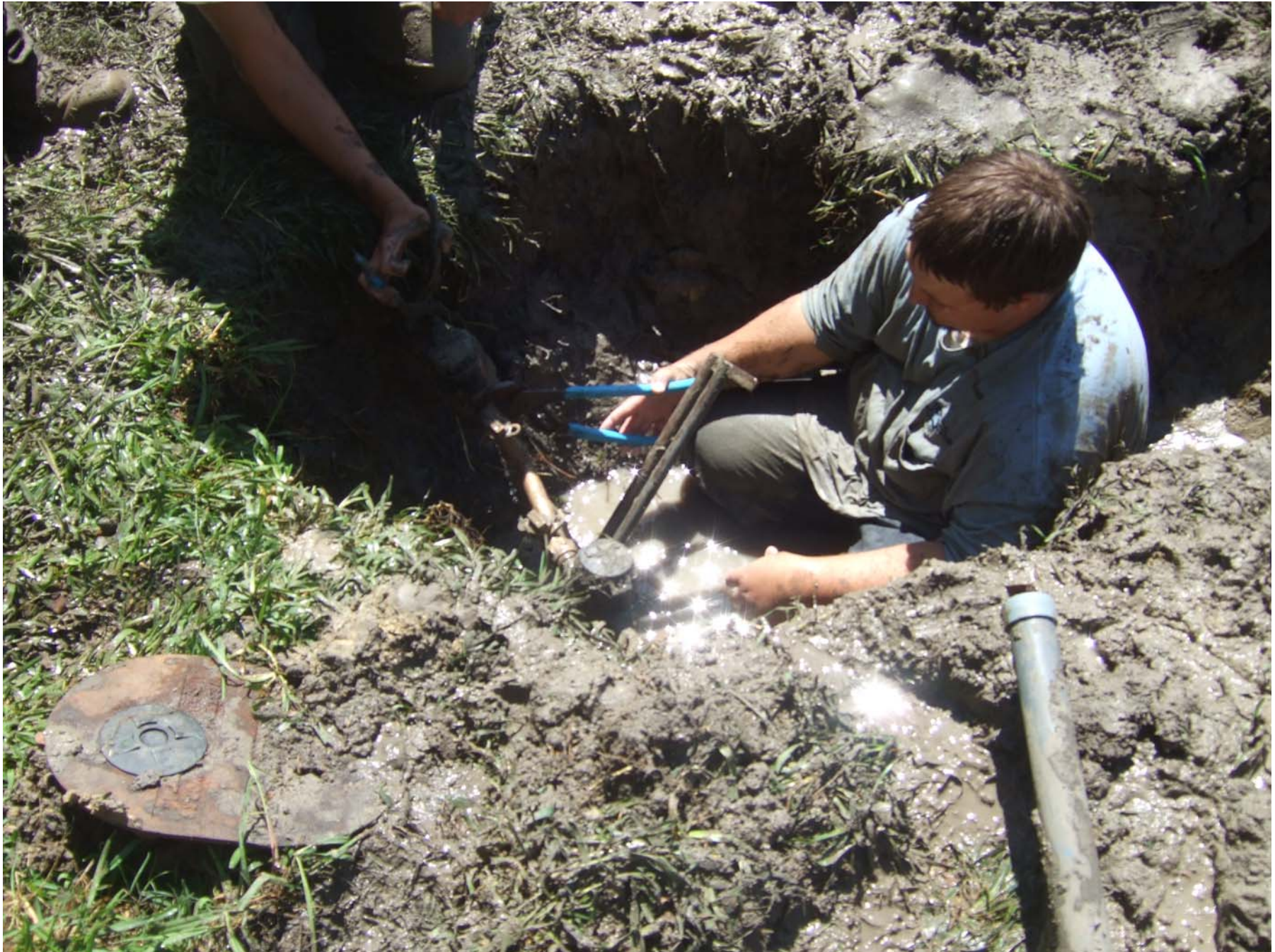
The problem: broken copper pipe and water still running
