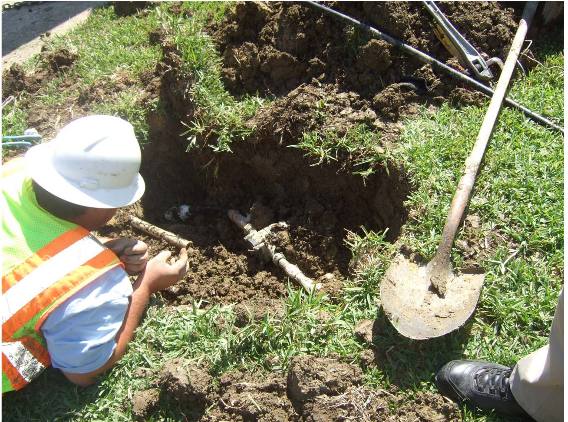
The final step: replace copper tubing with HDPE pipe using FloPlast CTS Fitting
