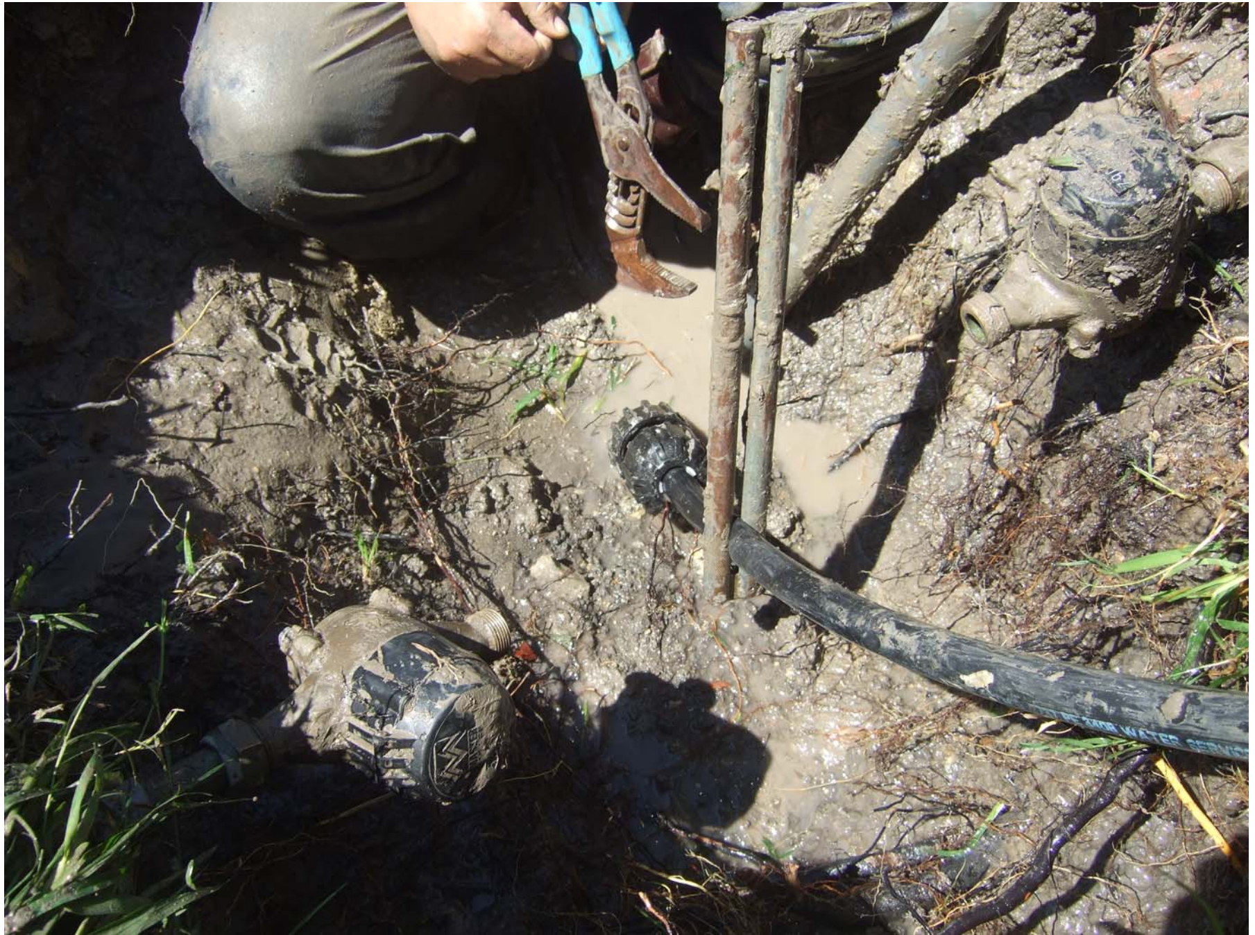
The solution: replace copper tubing with HDPE pipe using FloPlast Universal fittings. Copper on one end and new CTS size HDPE on the other. Installation took place while water was still running!
